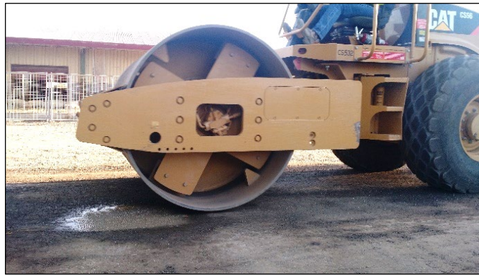
Figure 8.4: Checks for deformation between drum and FDR-C layer during microcracking. (Note vibration ripples on water.)
