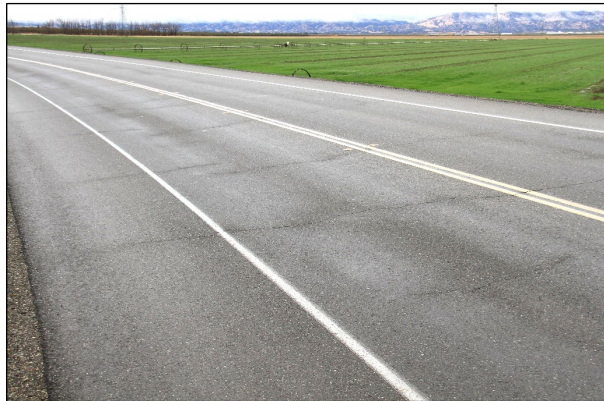
Figure 1.1: Reflected shrinkage cracks on an FDR-C pavement seven years after construction.
