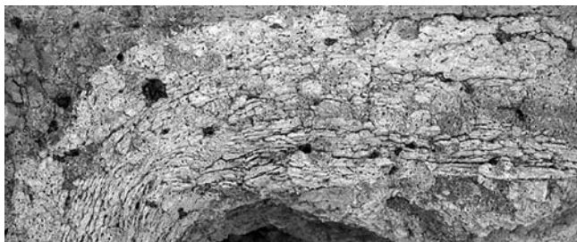
Figure 5.102. Photograph showing the thickness of the combined layers of wall plaster in the northeast corner of Space 87.
