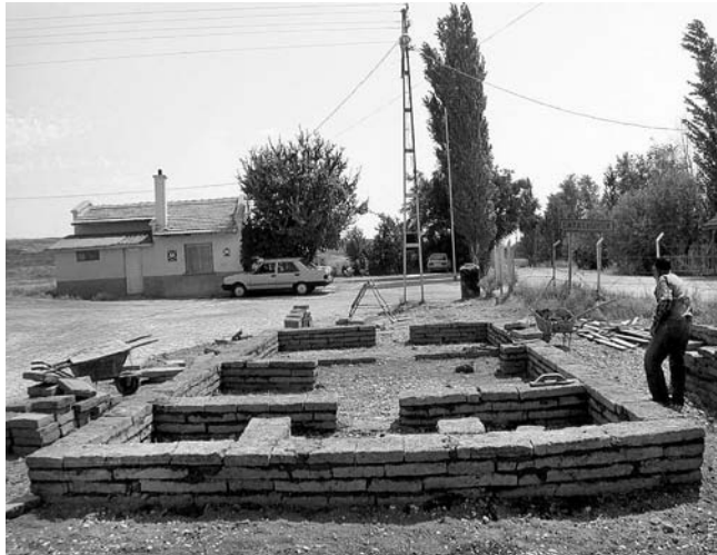
Figure 22.10. House construction: plan of the house and the initial courses of brick and mortar.
