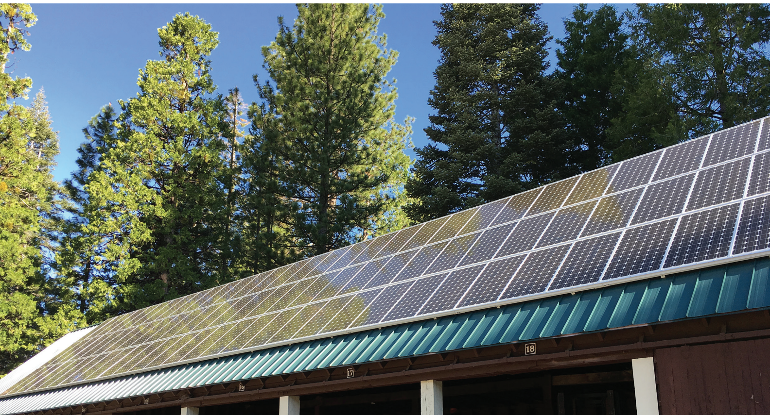
Rooftop solar panels, Lassen Volcanic National Park, California, USA. PATRICK GONZALEZ
