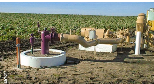
The recycling facility provides 65% of the water delivered to growers in the MCWRP area.
